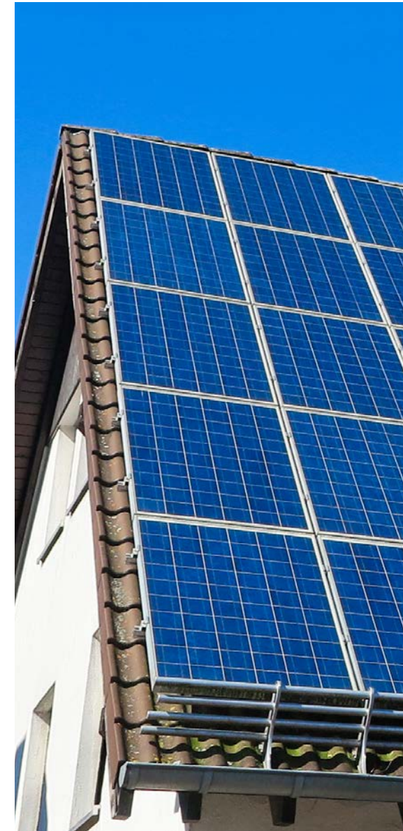
One of the services offered by Aecon's Green Home Energy Services group is solar PV panel installation
